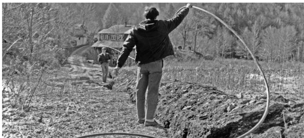
Grassroots activism: Student workers from Neighborhood Youth Corps lay a water line in North Carolina's Blevins Creek community in the mid-1960s.
